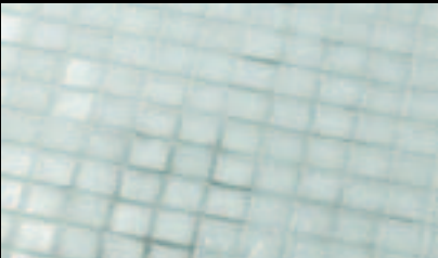
Often unhygienic: Grouted shower surface
